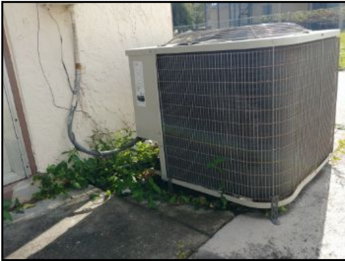
AC compressor- north
