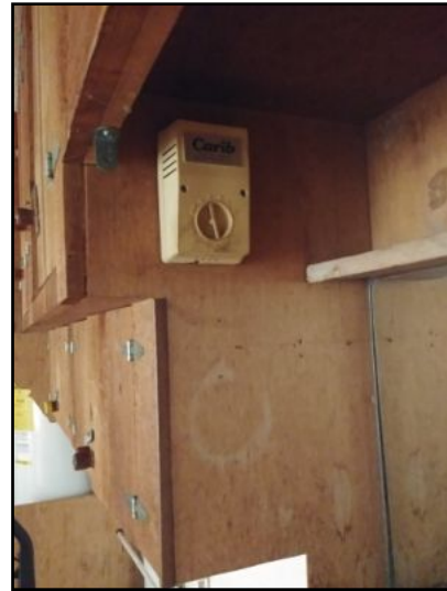
Fan control in garage
