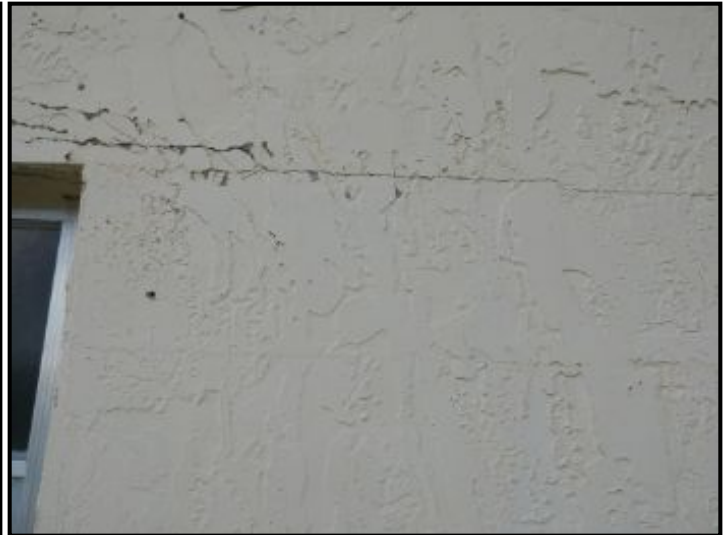
Cracks in stucco- north
