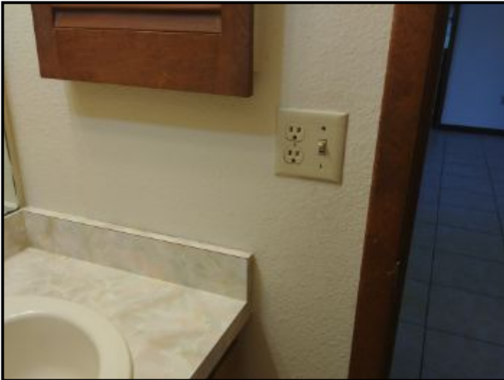
NO GFCI in hall bath
