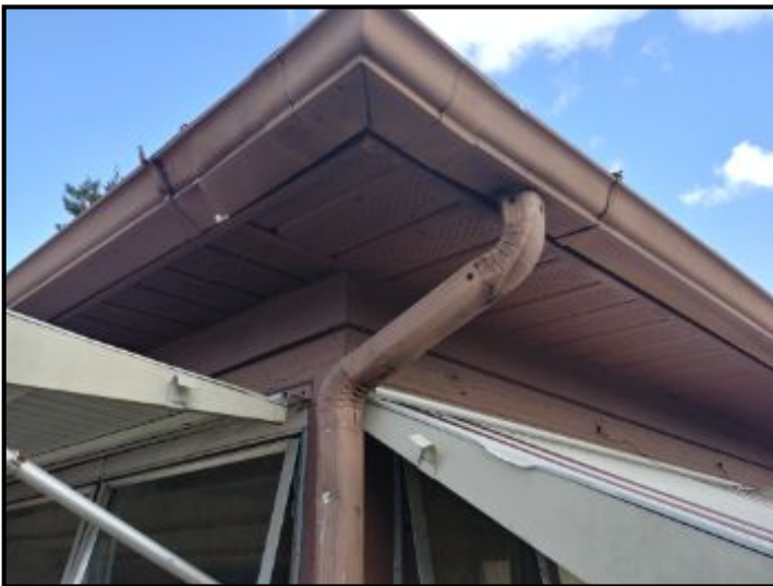
Loose gutter and leader- rear patio
