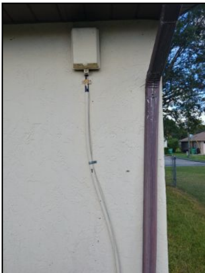
Alarm box rear
