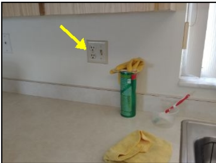
No GFCI in kitchen area
