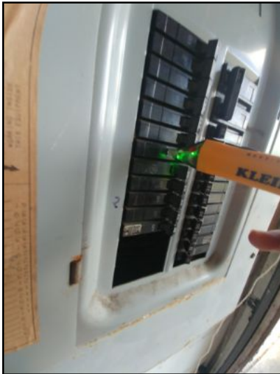
Test ok on some breakers
