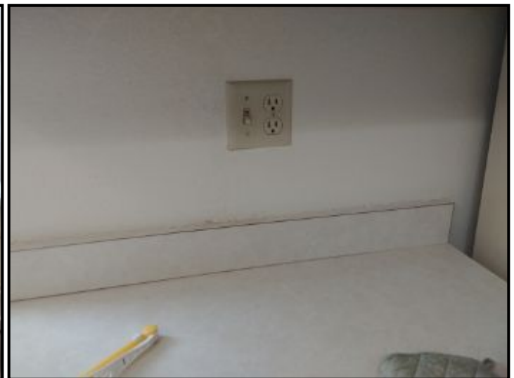
No GFCI at kitchen counter
