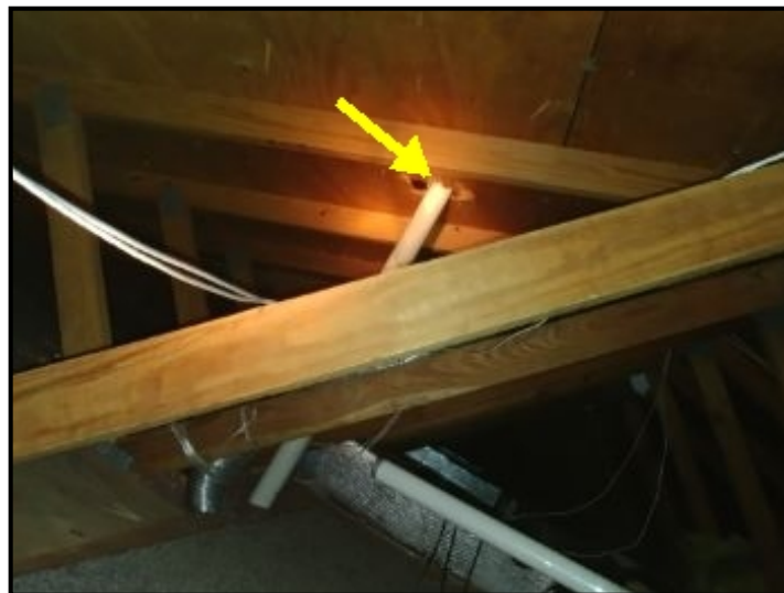
Large hole through roof pvc vent pipe
