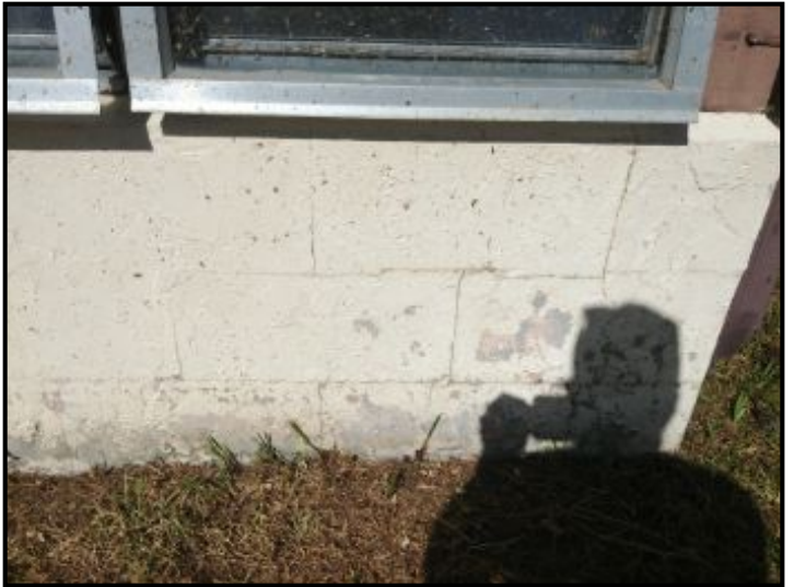
Cracks in block patio outside
