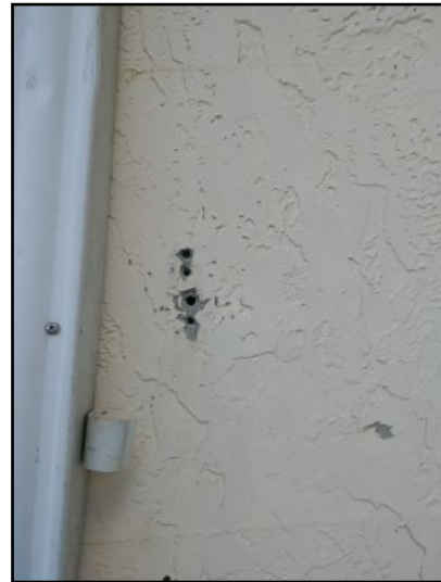
Holes in stucco and block- north
