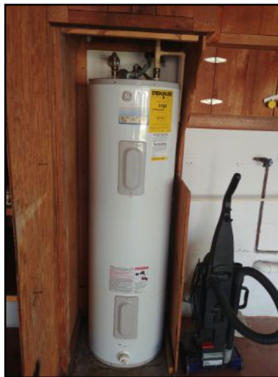
Water heater in garage
