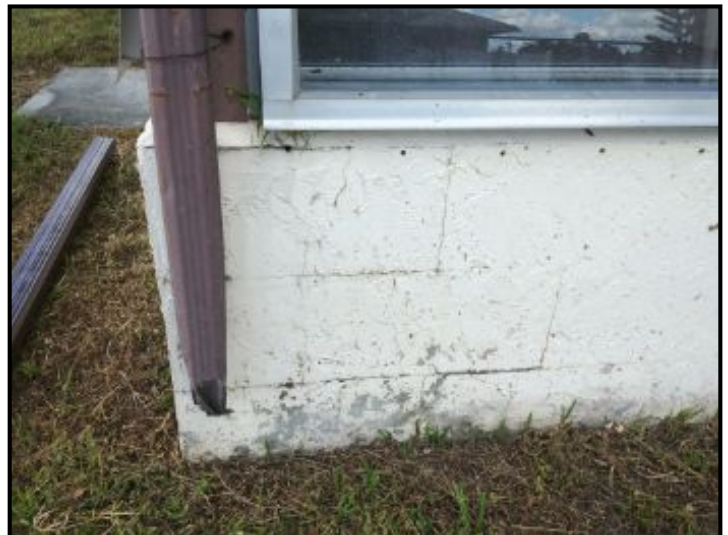
Cracks in block/crushed leader/missing elbow
