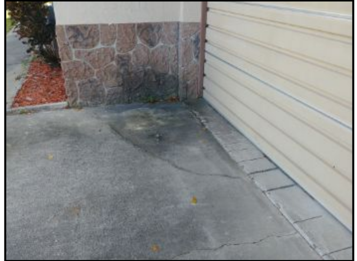
Improper slope due to cracks and back pitch
