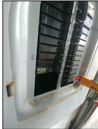
Voltage noted at panel breaker
