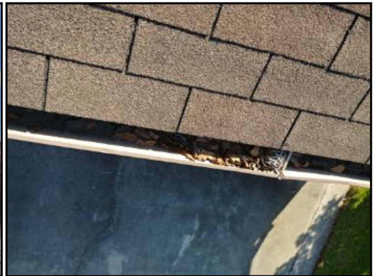
Leaves clogging gutter
