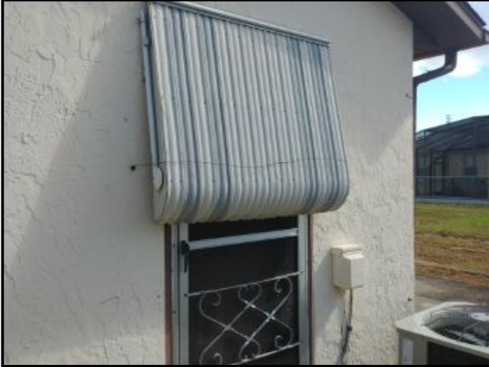
Awning blocking exit
