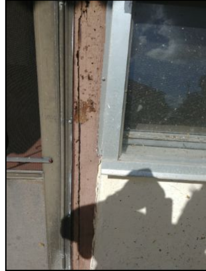
Wood at screen door extreme wear - rear
