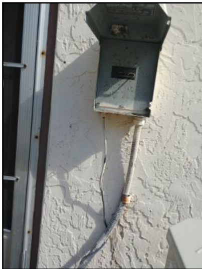
Outside breaker for AC
