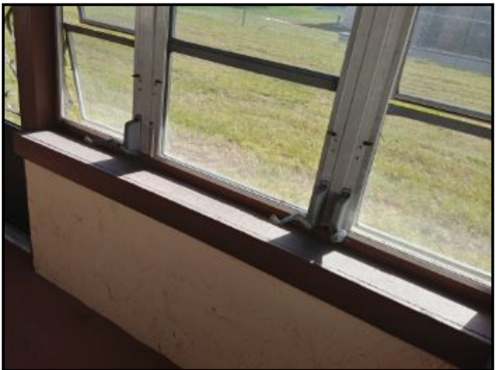
Patio awning windows
