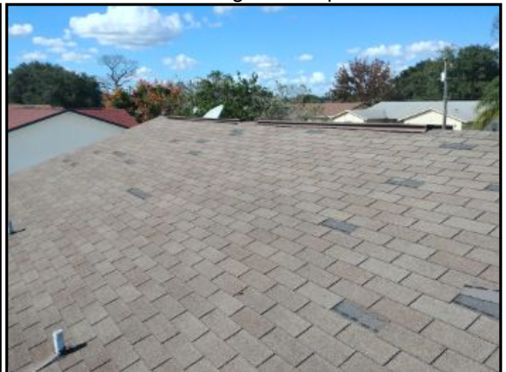
Broken shingles- west
