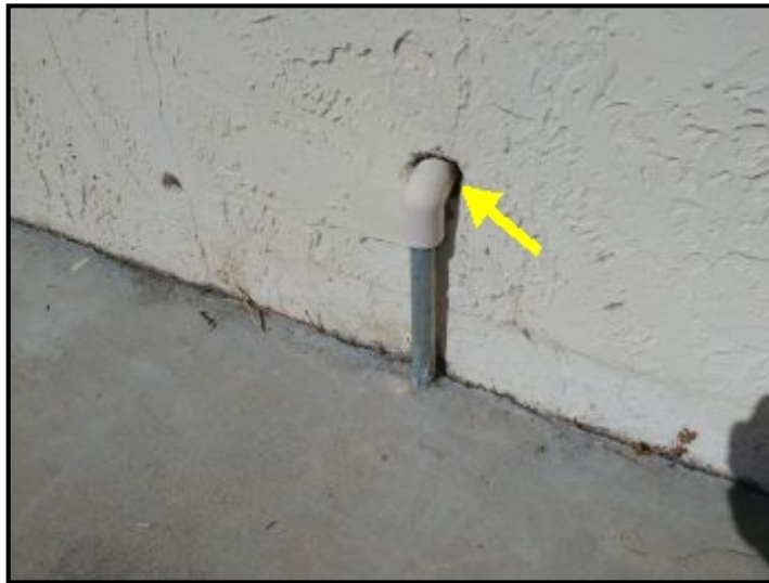
Needs sealing into house
