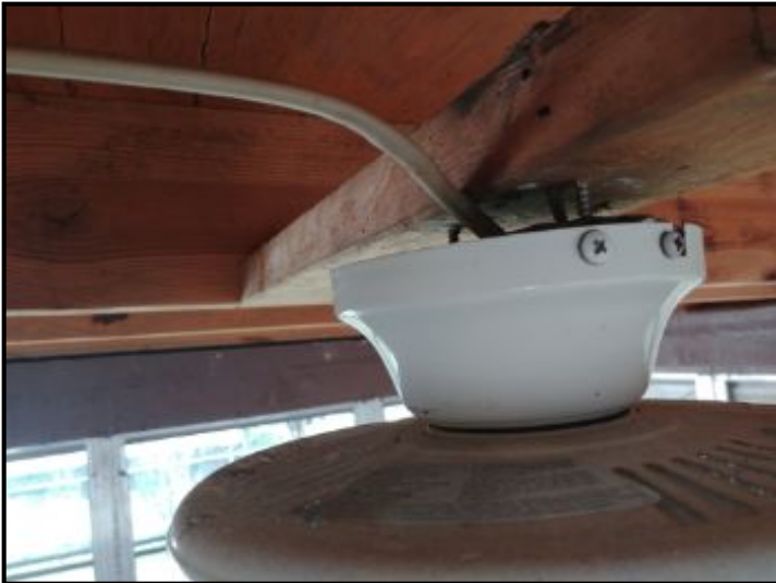
Missing mounting box
