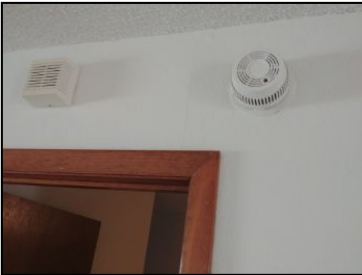
Living Room smoke detector/alarm box
