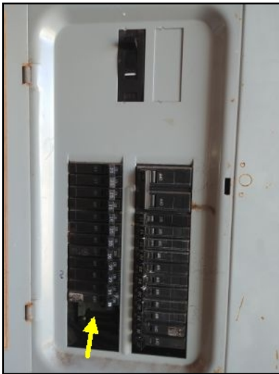
Open Breaker spaces in panel
