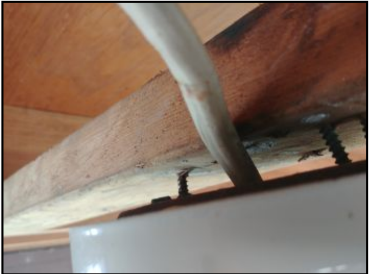
Patio fan improper mounting
