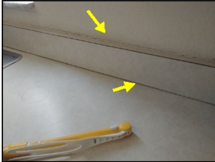
Gaps in back splash and to wall
