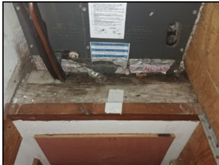
Signs of prior water at AC handler
