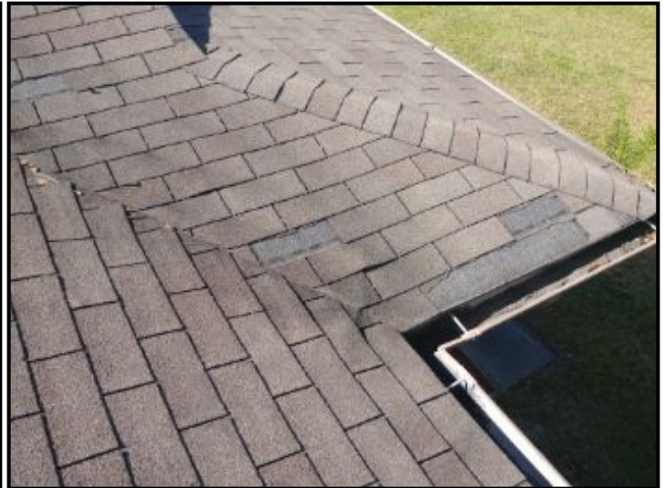
Missing shingles at valley
