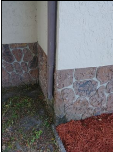
Gutter discharging against foundation and bed
