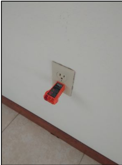
LR outlet lower not working
