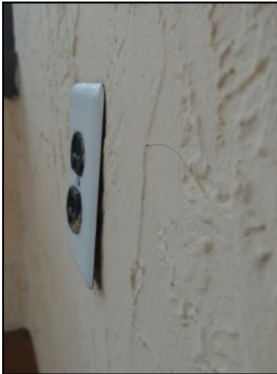
Patio switch plate loose
