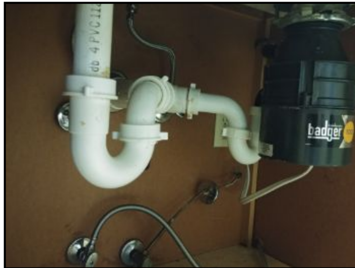
Disposal and drain- kitchen sink
