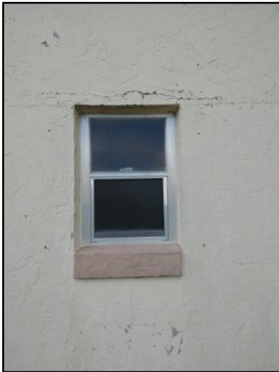
Cracks over window- north
