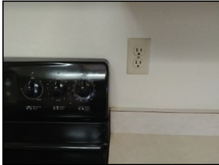
No GFCI in kitchen area
