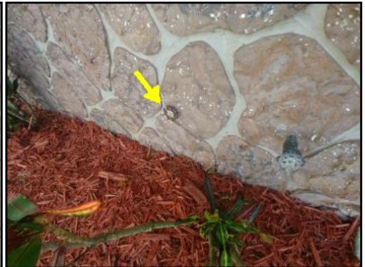
Front and MAIN water shut off
