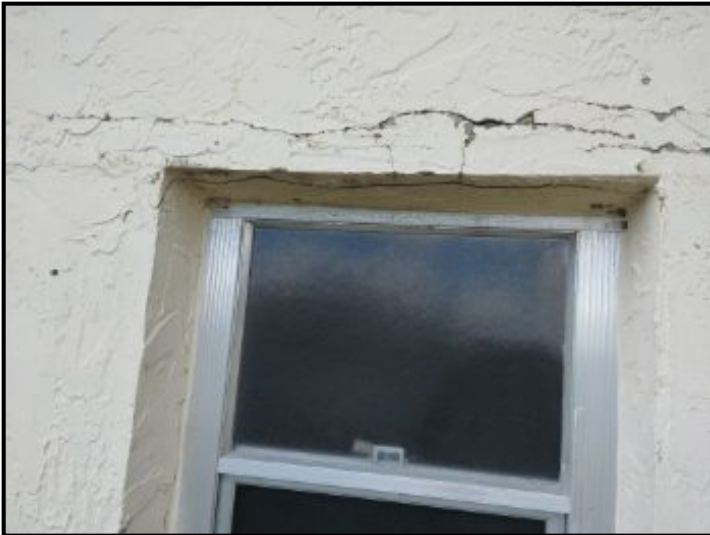
Extreme cracks over master bath window- north
