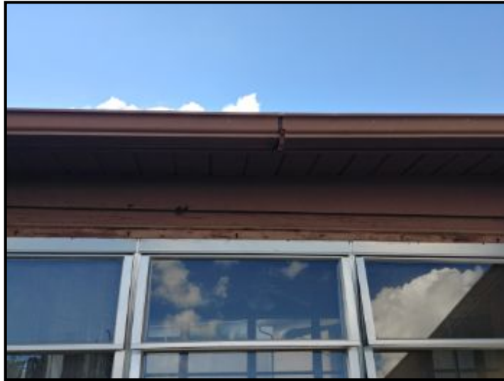
Wood worn and pitted- rear patio
