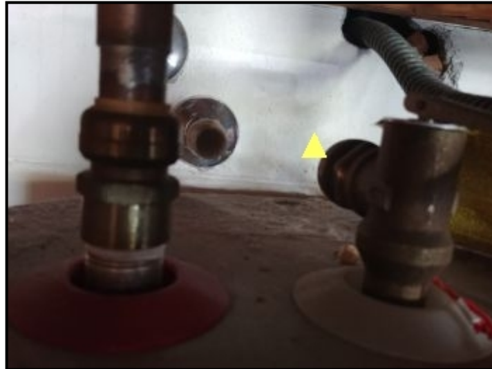
Missing TPR valve
