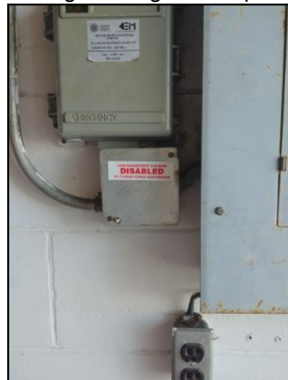
Electrical utility panel in garage
