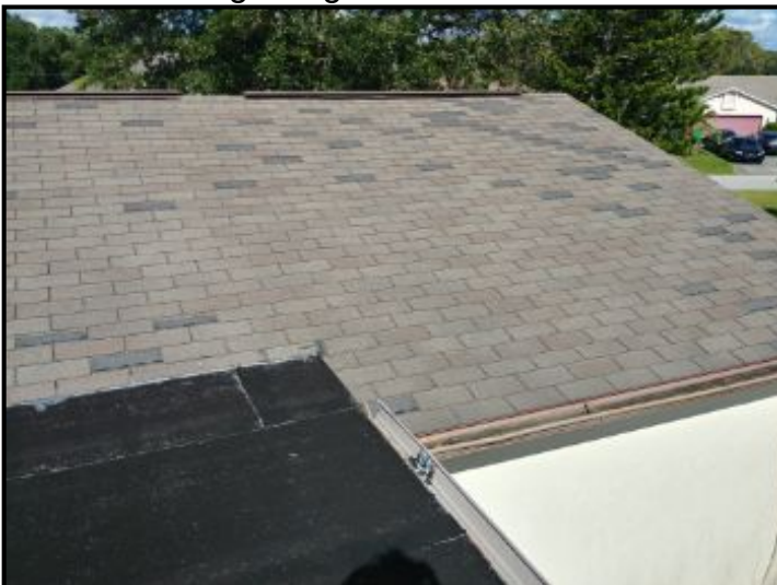
Missing/broken shingles- west
