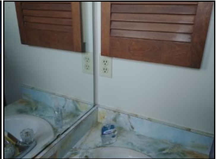
No GFCI in master bath
