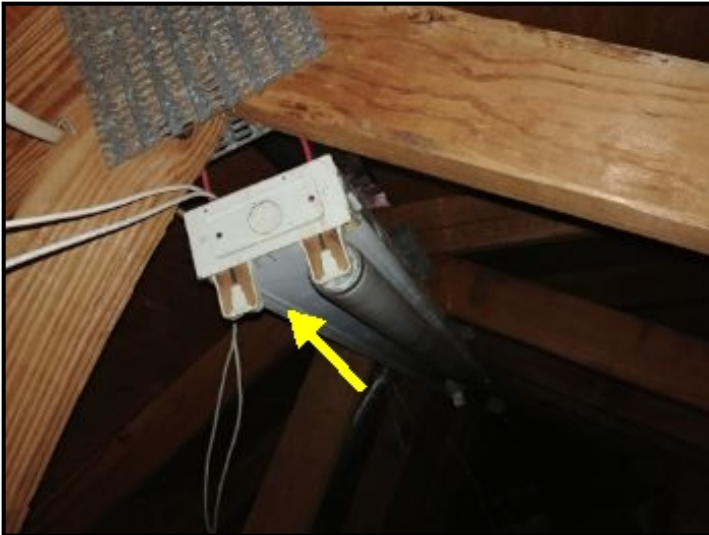
Missing bulb/ unsecure wiring
