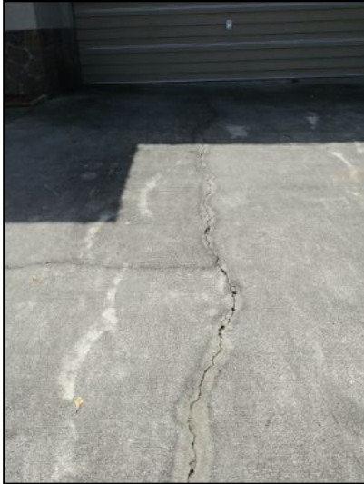
Cracks in driveway
