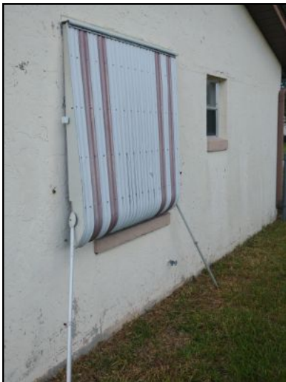
Unsecured awning- north
