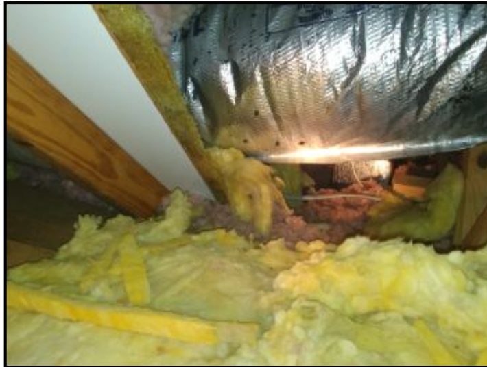
Attic insulation and AC duct
