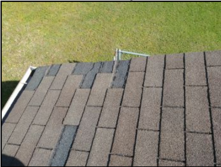
Missing shingles at rake and eaves
