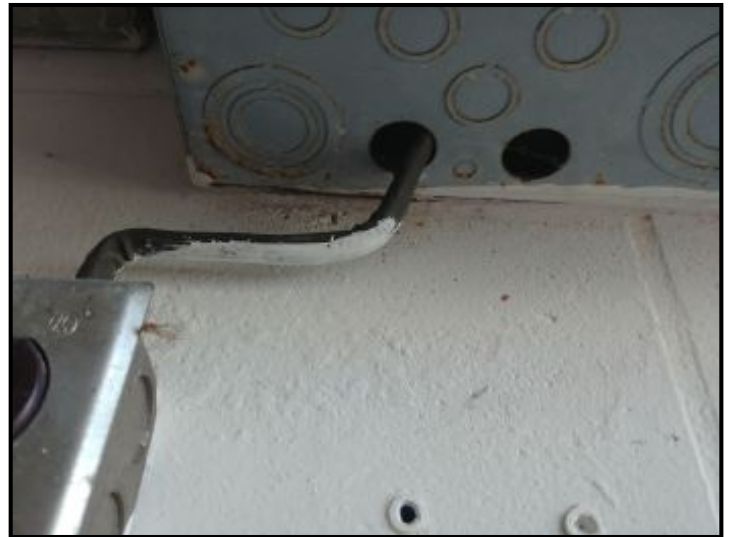
Missing bushings under panel
