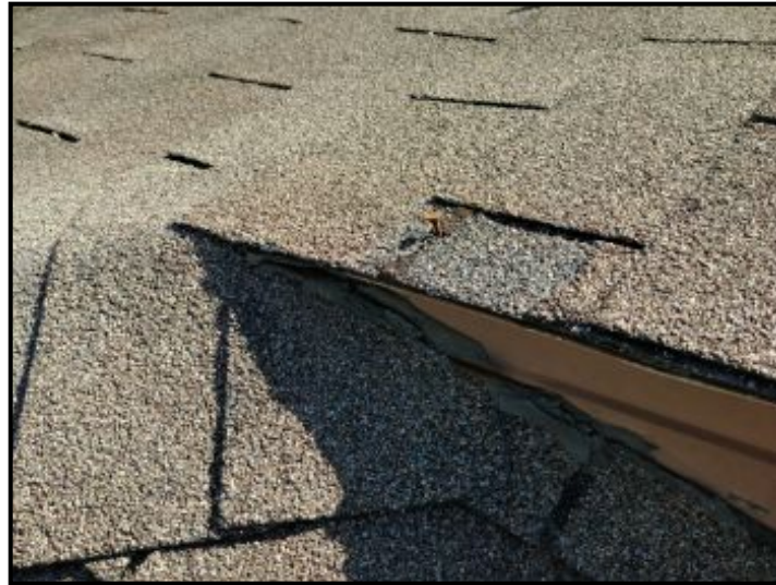
Flashing not visible
